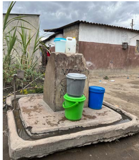
Figure 5: A broken down communal water tap in Chawama of Lusaka
